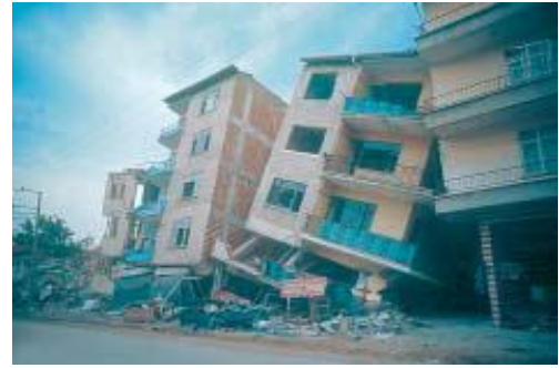
Sway mechanisms are often inevitable with soft storey ground floors (Izmit, Turkey 1999).
